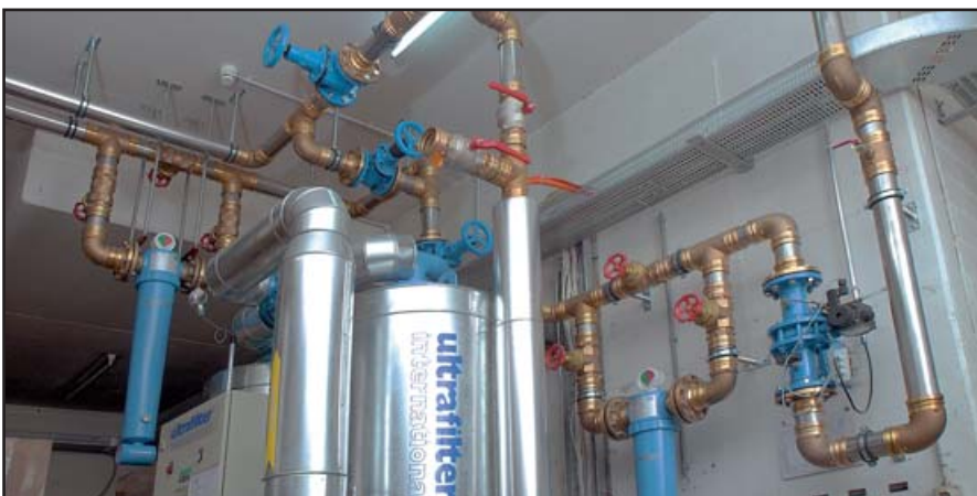
Ultrafilter and dehumidifier unit of the compressed air system with exhaust pipes in Optipress XL Ø 89 mm
