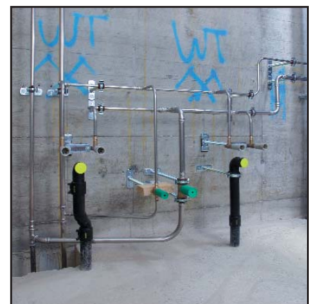
Sturdy installation down to the taps
