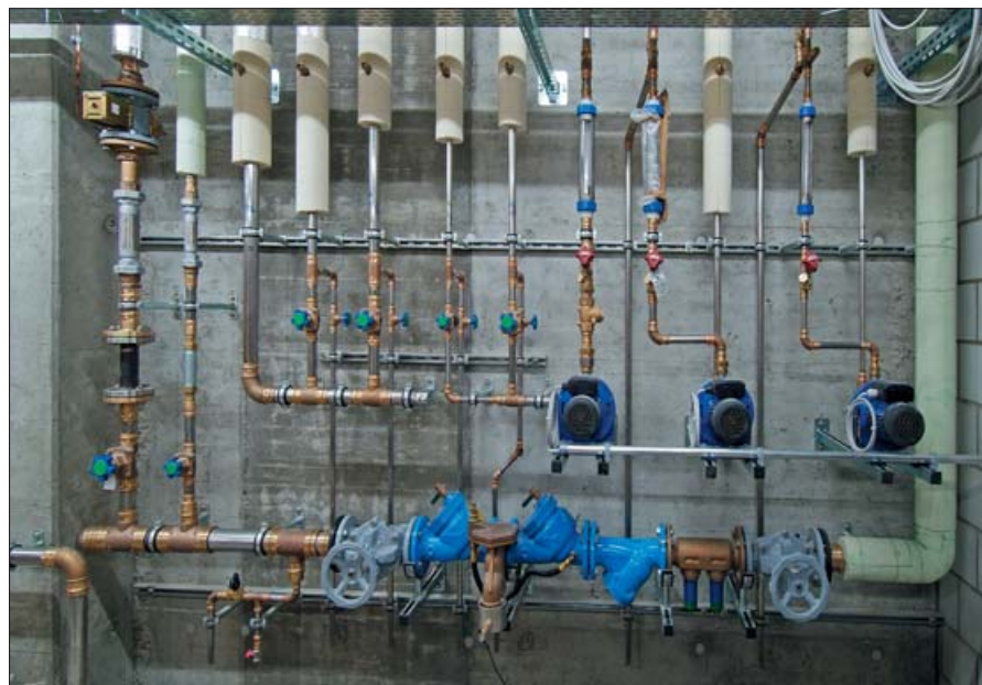
The hot water distribution with feeders to the Coop Megastore refrigerating plant
