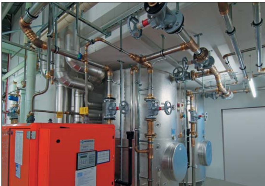
The water heating system for the sports facilities incl. gymnasium
