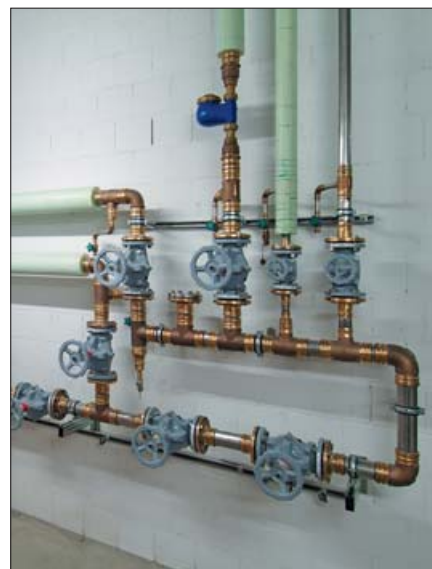
The cold water distribution system for the sports facilities incl. gymnasium
