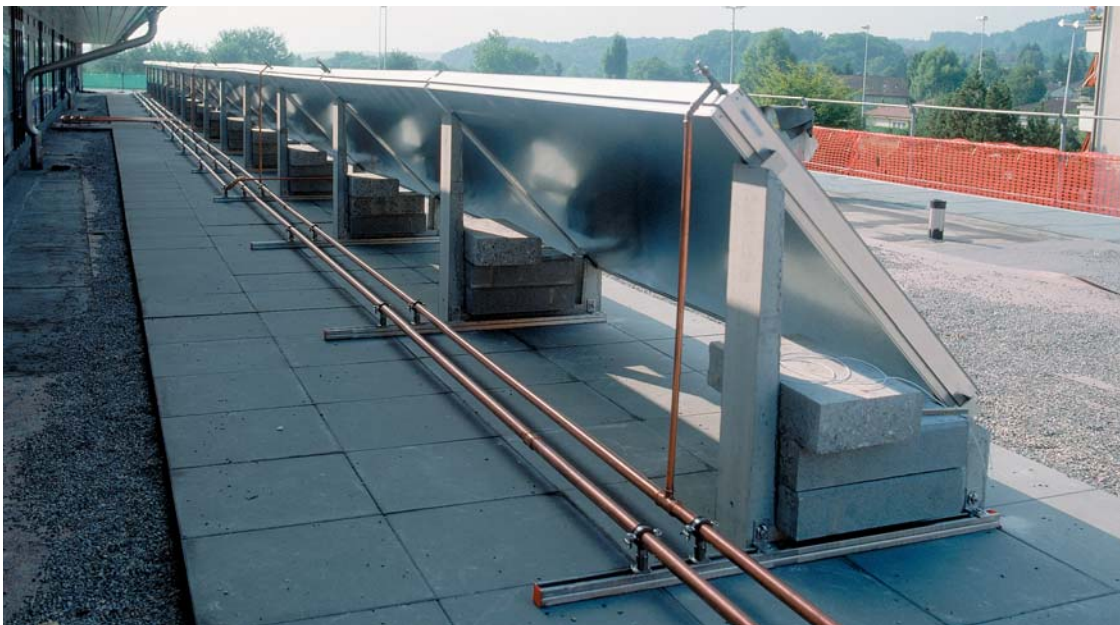
15 solar collectors with copper pipework using the Cupress installation system (shown prior to lagging).
