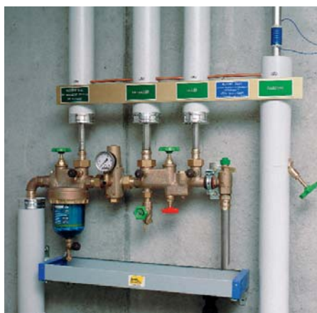
This central water supply unit has been installed in every house and it meets every requirement.
