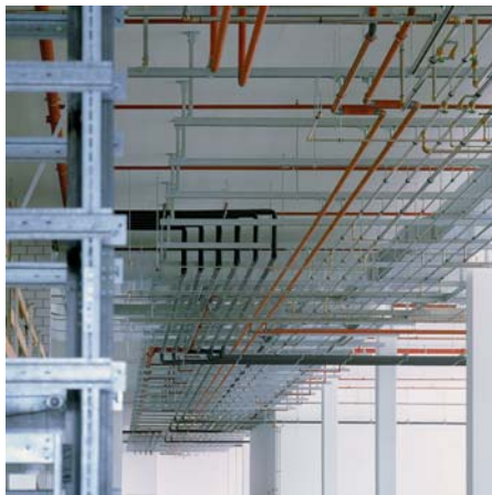
The various water-supply networks (before lagging).
